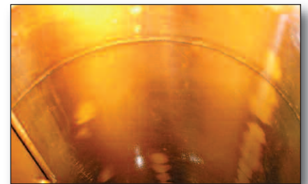
Filter housing internals coated with varnish
